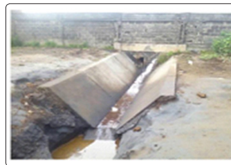
Figure 3a: Discharge from depot into unlined pit
